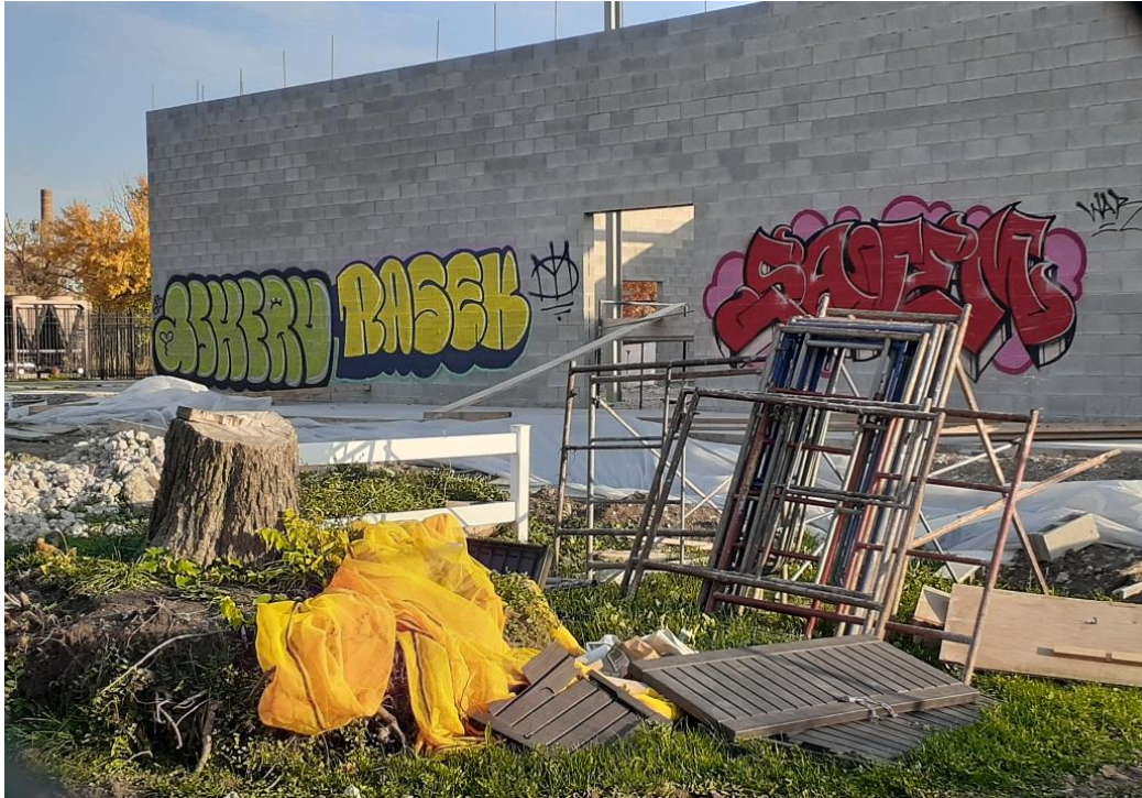
Figure 5 Graffiti on unsecured construction site; evidence of stump of mature tree removed without permit; photo taken 12/09/2022; Source: Kurt Gippert
