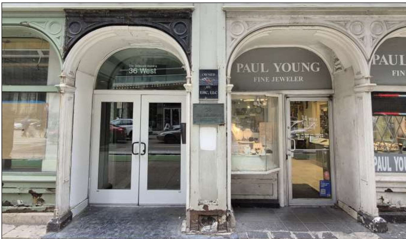
Deterioration at ground floor entry, Delaware Building, 1872-1874, Wheelock & Thomas, 36 W. Randolph Street. Photo credit: Ward Miller
