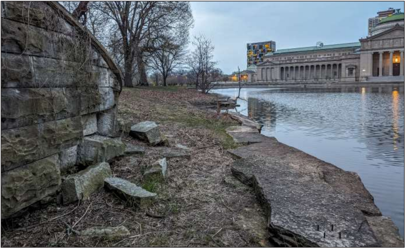
Fallen stones at Clarence Darrow Memorial Bridge / Columbia Bridge, 1880, Burnham & Root, 1766 Columbia Drive. Photo credit: Eric Allix Rogers
