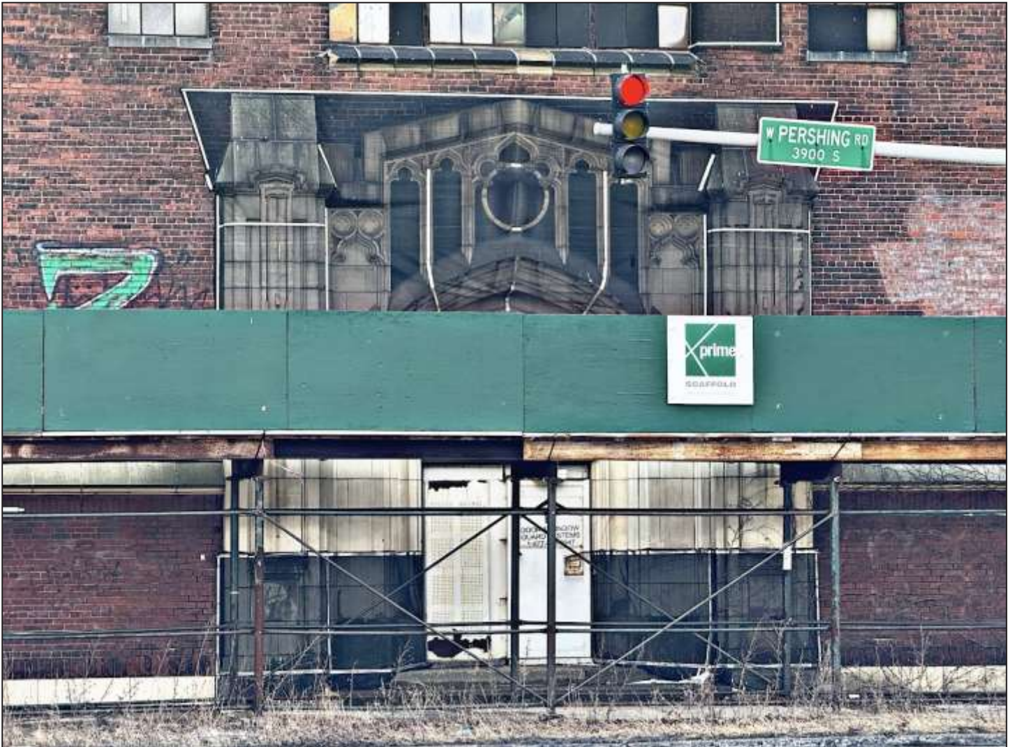
Deferred maintenance and scaffolding visible at main entry to Central Manufacturing District Clock Tower Building, 1917, Samuel Scott Joy, 2000 W. Pershing Road. Photo credit: Cristen Brown
