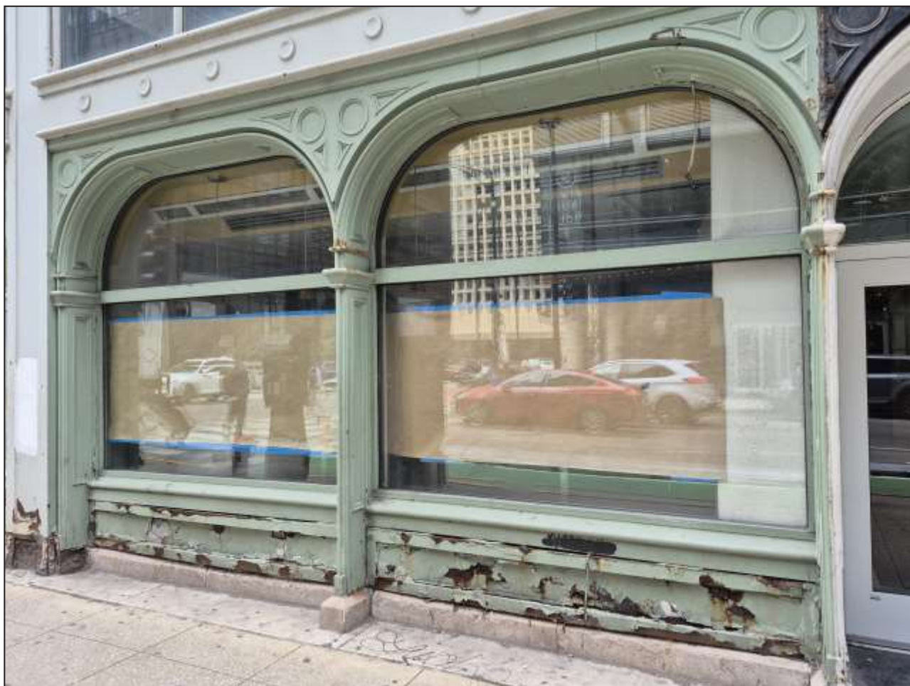
Deteriorated storefronts, Delaware Building, 1872-1874, Wheelock & Thomas, 36 W. Randolph Street. Photo credit: Ward Miller
