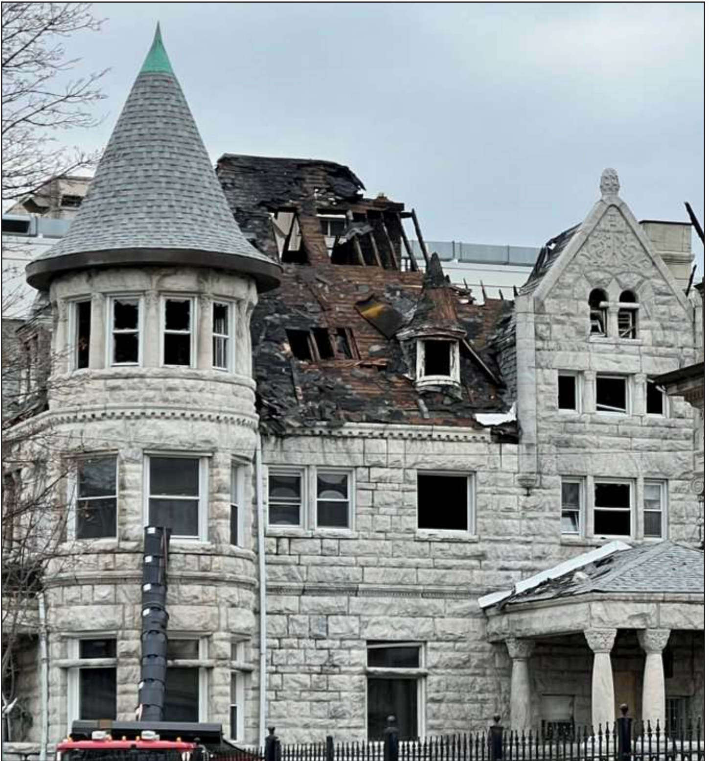
Aftermath of the 2023 fire at the Swift-Morris Mansion, 1892, Willett & Pashley, 4500 S. Michigan Avenue. Photo credit: Debbie Mercer
