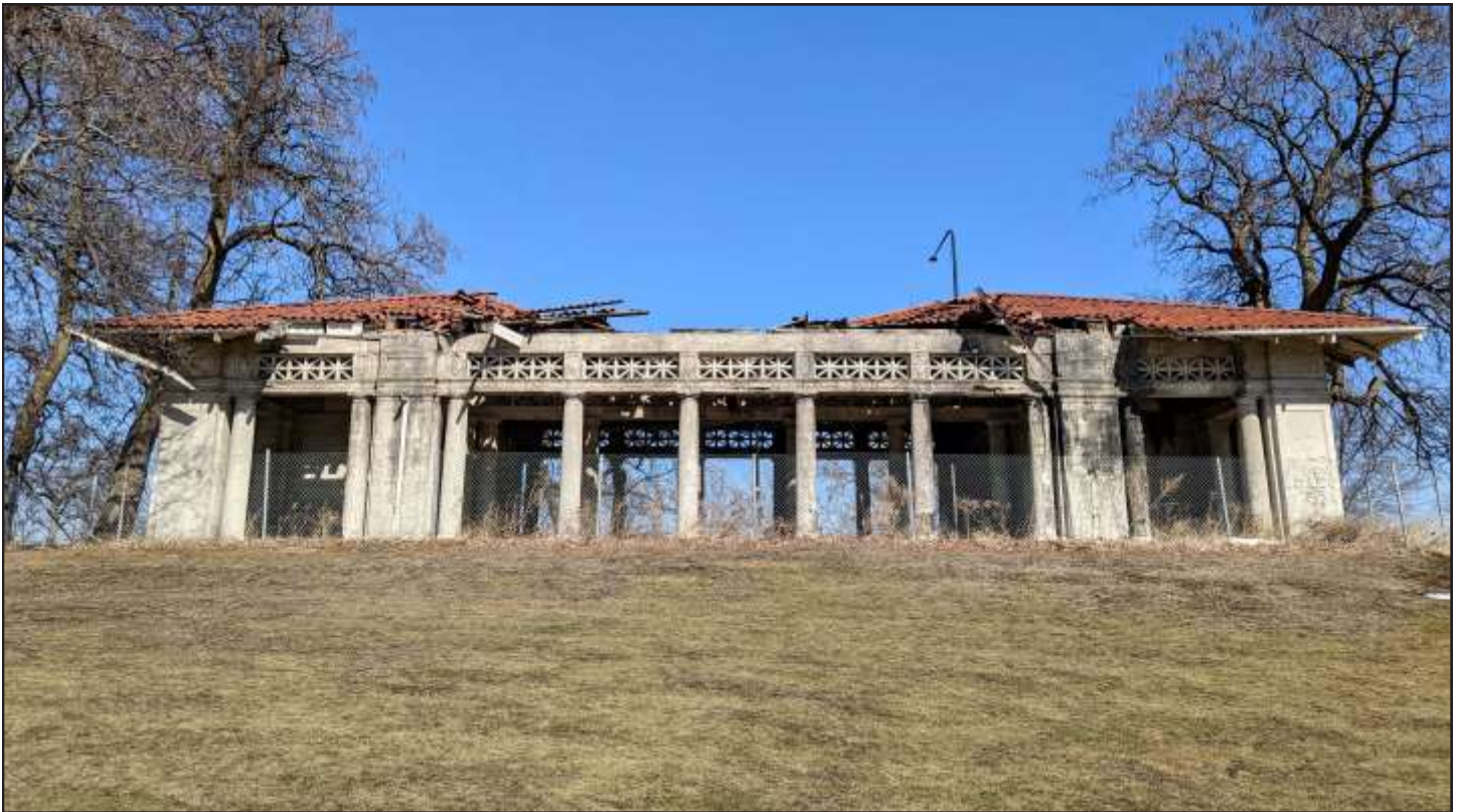
Crumbling Burnham-Designed Comfort Station in Jackson Park © Eric Allix Rogers
