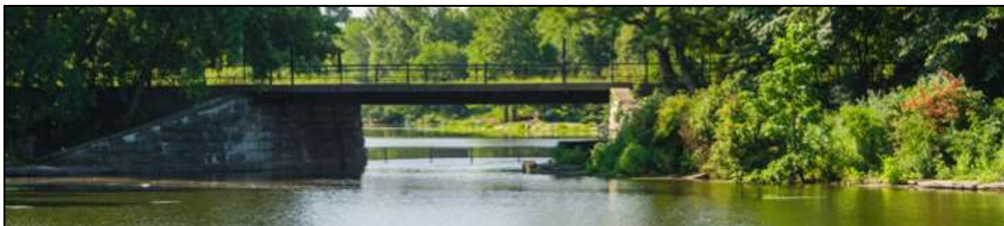
Hayes Drive Bridge, Music Court Bridge, Columbia/Clarence Darrow Bridge in Jackson Park all in need of repair © Eric Allix Rogers
