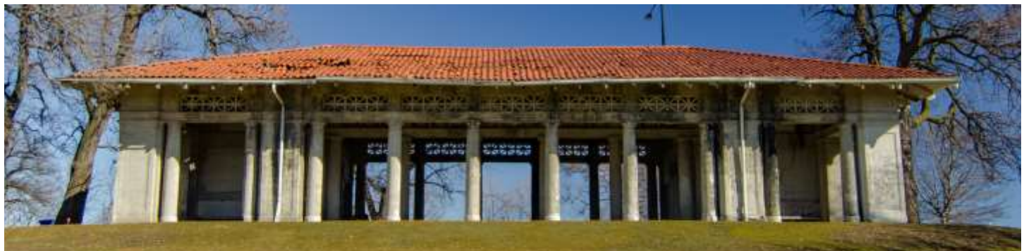
Jackson Park Comfort Station on South Shore Dr. near 67th St. by D.H. Burnham with evidence of deferred maintenance © Eric Allix Rogers
