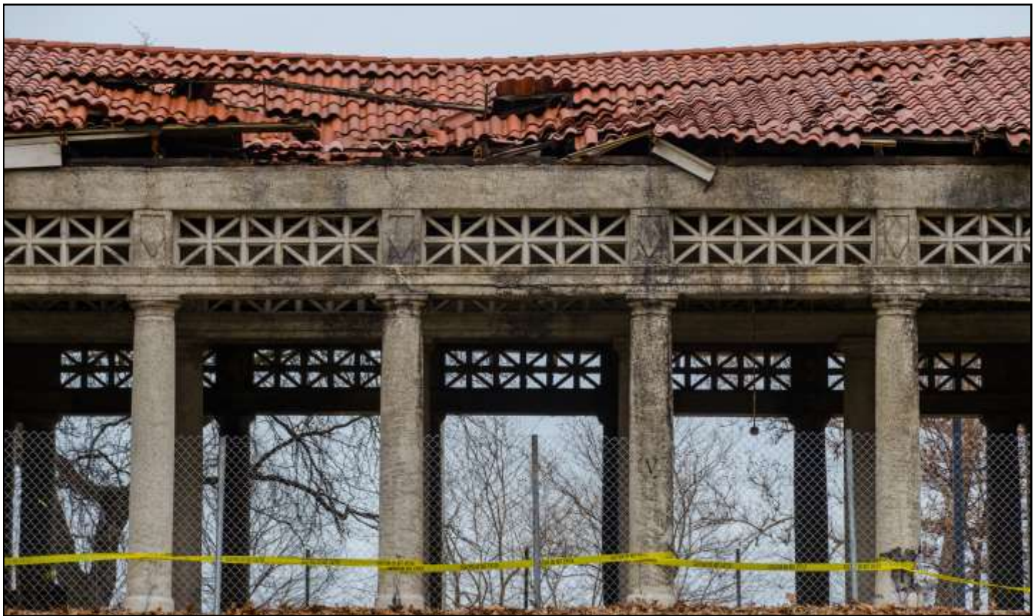
Jackson Park Comfort Station on South Shore Dr. near 67th St. by D.H. Burnham with evidence of deferred maintenance © Eric Allix Rogers
